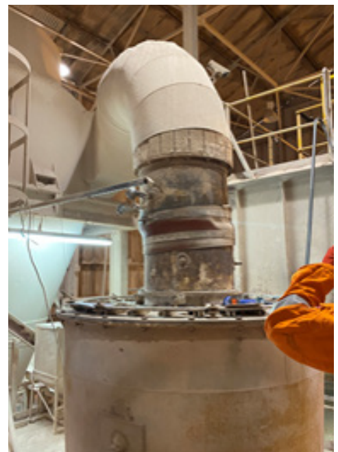
Figure 1: Mill and Classifier BEFORE overhaul. Note the confined workspace.
