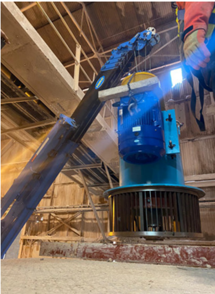
Figure 2: New VBC installation.
